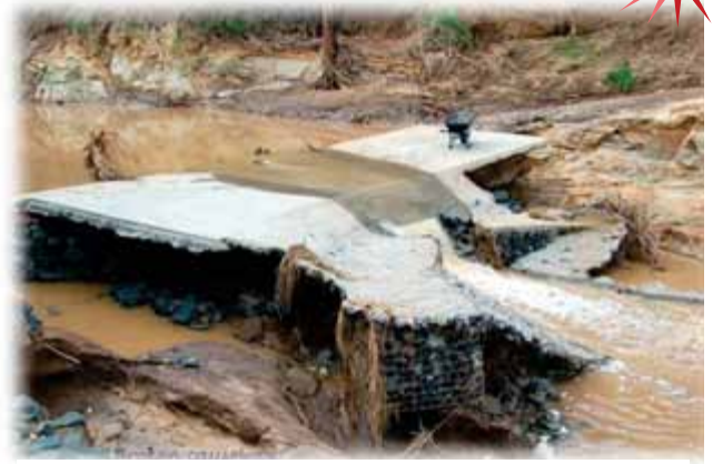
Broken causeway to the boarding kennel
